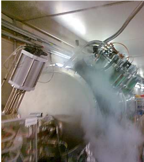
Figure 3. IDs: The superconducting wiggler as is being filled with liquid helium through a refilling line. Refilling can take place from outside the tunnel without affecting the performance of the machine. Restricted access to tunnel is only needed to open and close the valves.
